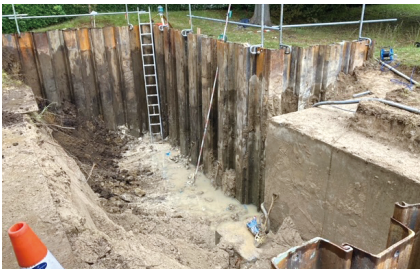
Excavation and removal of contaminated soil (former Advanced Materials Research Laboratory of Toyo Ink SC Holdings Co., Ltd.)
